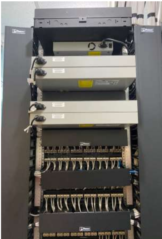
Figure 2 Front view of the Network Rack used for our experiment
