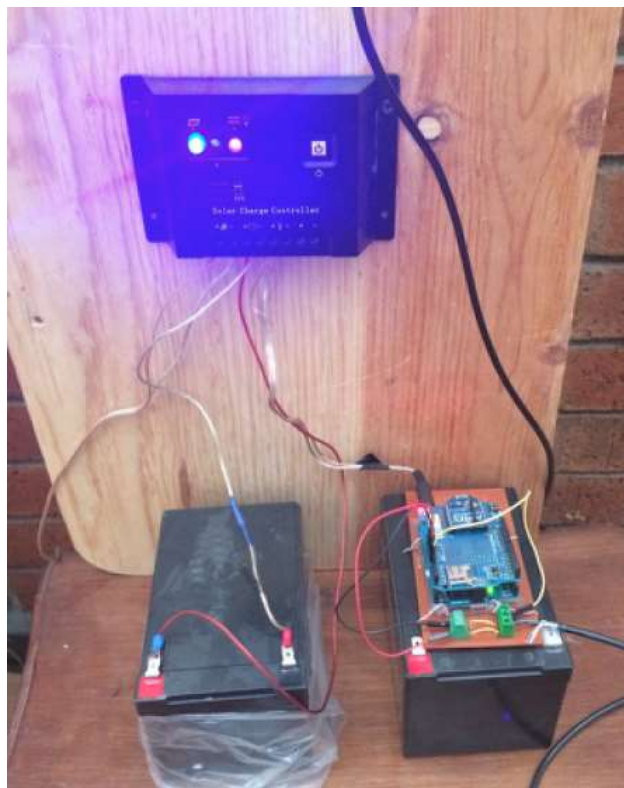
Figura 2 Transmitter. Notice an Arduino Uno microcontroller, powered by power from a solar cell. See the cable that goes up, corresponding to the Vaisala probe, which does the temperature measurement.
