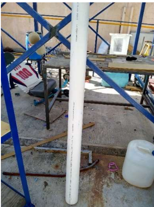
Figure 3 Sanitary PVC Pipe Own Elaboration
