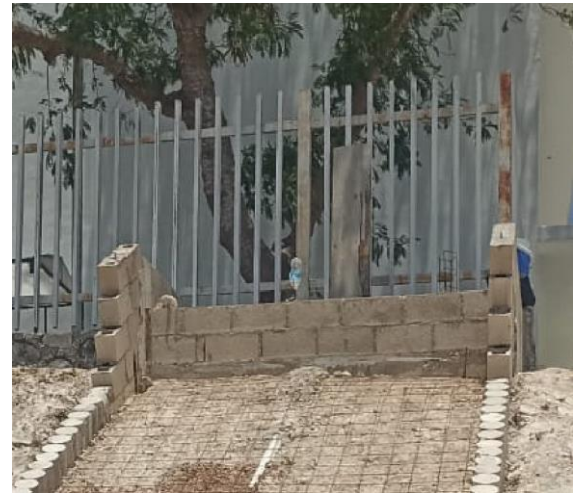
Figure 3 Bottom tank construction. a) Laying of electro-welded mesh, b) Construction of walls
