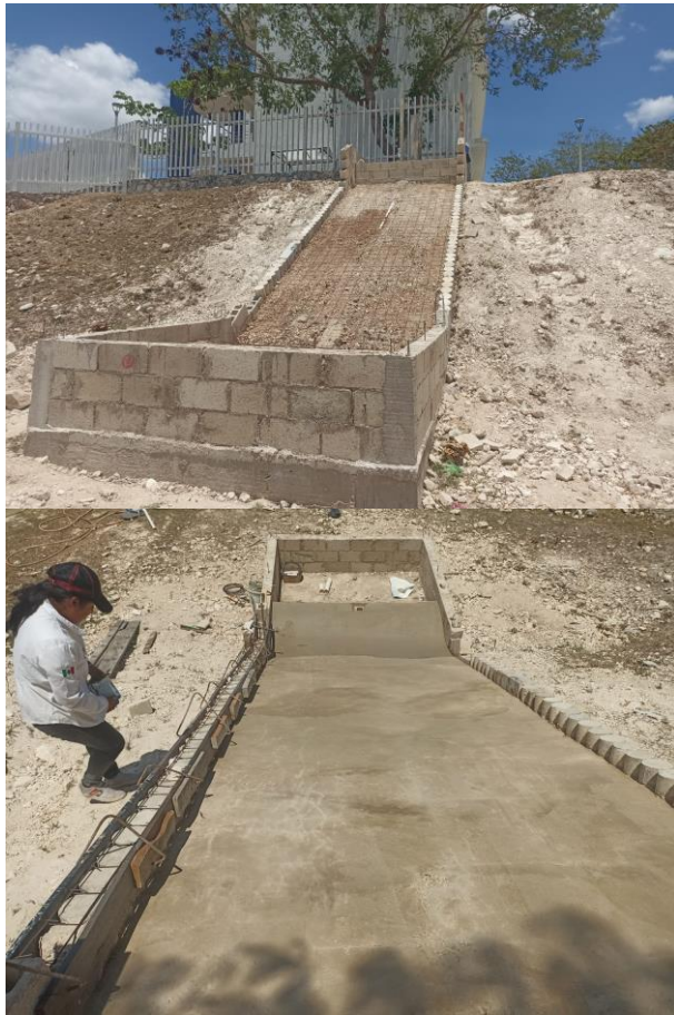
Figure 5 Screen construction. a) Laying of electro-welded mesh, b) Casting Source: own elaboration
