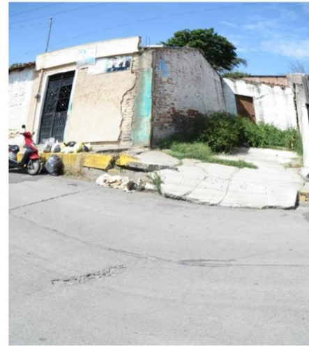
Figure 5 Damaged houses in Cd. Guzmán Source: (Photo from Maciel-Flores archive)
