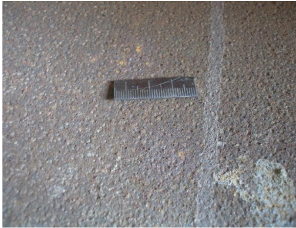
Figure 5 The image shows corrosion pitting inside the tube. (The layer of red corrosion products was removed from the surface) Source: Own work
