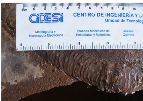
Figure 3 The image shows the right area of the crack. There is seen the change in crack growth from the weld toe to the body of the pipe
