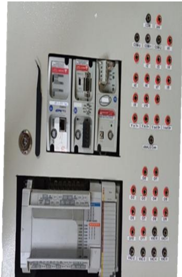
Figure 7 Electrical panel for PLC Micrologix 1500. Source: Own elaboration, 2024
