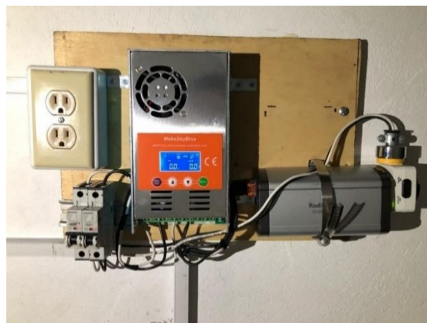
Figure 6 Controller connected Source: Own elaboration
