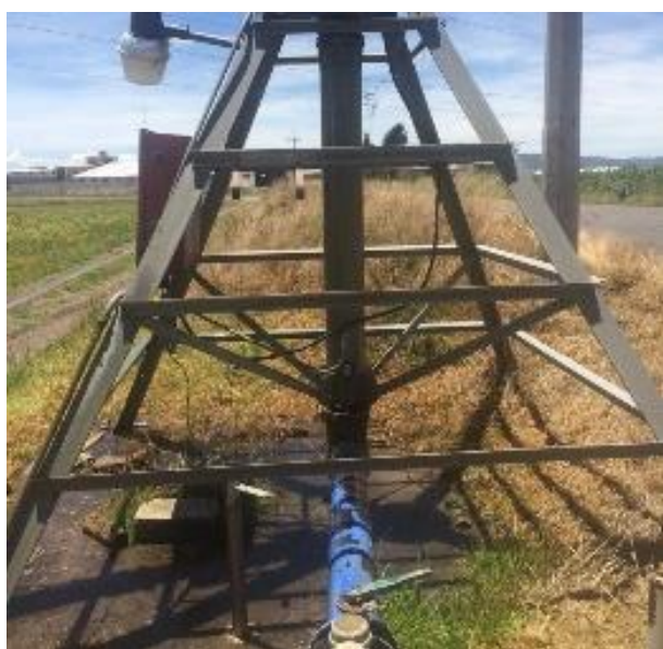
Figure 8 Main pipe and stopcock
