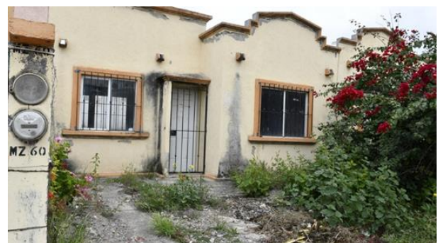
Figure 1 Cracking and moisture in the walls and slabs
