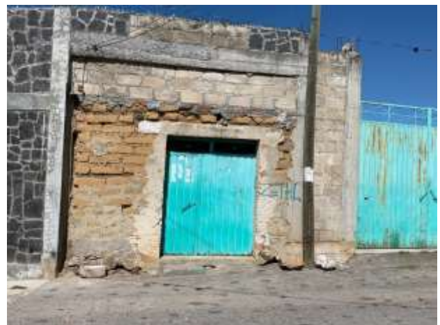
Figure 8 Adobe house with interventions using, heavy block, stone and the inclusion of columns, chains and beams that modify its configuration. Huaquechula, Puebla, 2017
