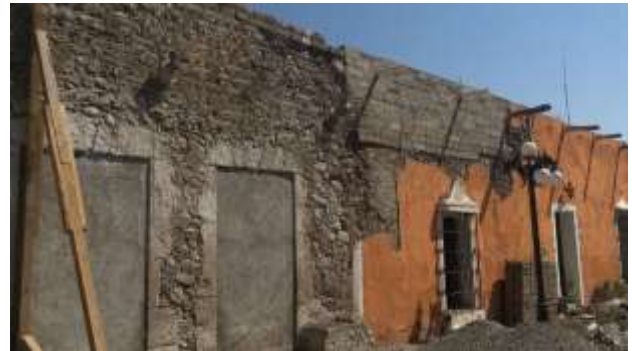
Figure 7 After the 2017 earthquake, the parapets came off in buildings classified as historical heritage, which is why different materials were used in the intervention. In the case of the house on the right, it was made of a parapet with hollow cement blocks, which is a material incompatible with adobe. Atlixco, Puebla, 2017
