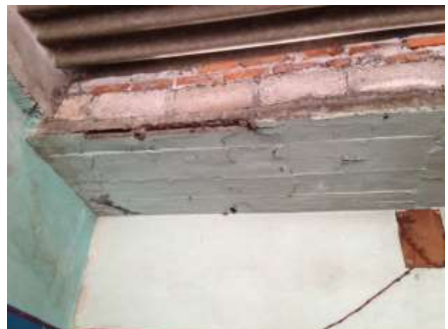
Figure 9 Adobe house in Chietla, the epicenter of the 2017 earthquake, where reinforced concrete slab was incorporated. Buap, 2017
