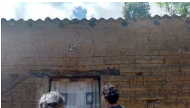
Figure 6 Door lintel damaged by weathering that affects its useful life in San Juan Bautista, Tochimilco, Puebla, 2017
