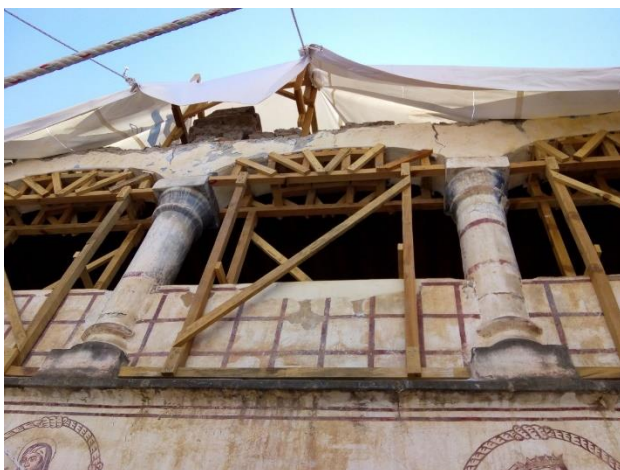
Figure 5 The courtyard of the convent has columns and lowered arches on the ground floor and upper floor. The arches of the upper floor were damaged during the 2017 earthquake and the shoring of the arches is shown in the image
