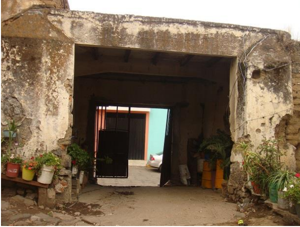
Figure 8 Access to the property, where the roof of beams and brick is observed Source: Vázquez, 2017
