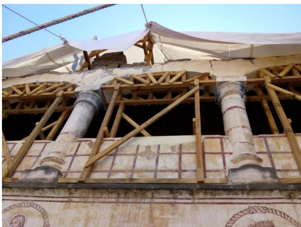
Figure 5 The courtyard of the convent has columns and lowered arches on the ground floor and upper floor. The arches of the upper floor were damaged during the 2017 earthquake and the shoring of the arches is shown in the image
