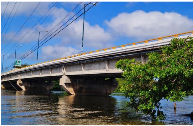
Figure 1 Photograph of the Champotón Bridge. Panoramic view of the bridge, from the north-south point Source: own (2019)
