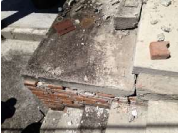
Figure 15 In several houses it was observed that the constructions of unconfined masonry were placed reinforced concrete roofs that caused separation between the slabs and compression in the walls
