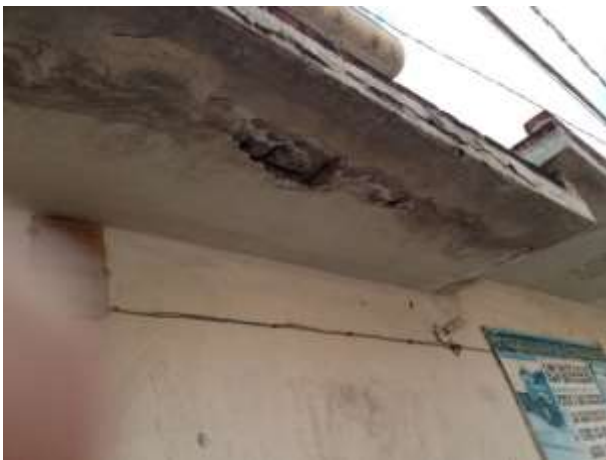
Figure 16 A common problem was that the eaves were too long and flexed causing cracks that moisture caused the degradation of the materials
