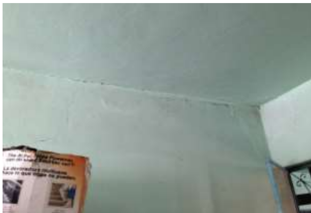
Figure 11 Unconfined walls, observed at the top of the wall, the separation of the wall with the roof Source: Faculty of Architecture BUAP, 2017
