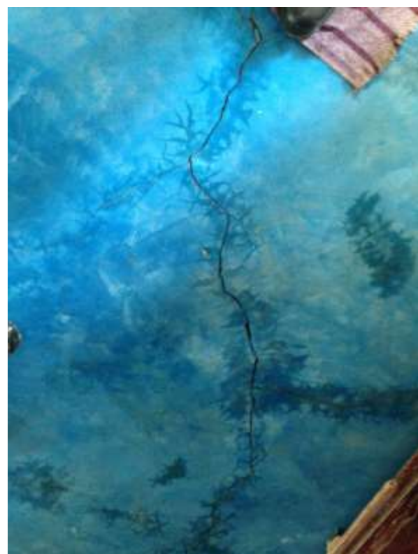
Figure 17 It was observed that there were already cracks produced by other earthquakes, in which the humidity caused more fissures than in the earthquake of 2017 were evidenced
