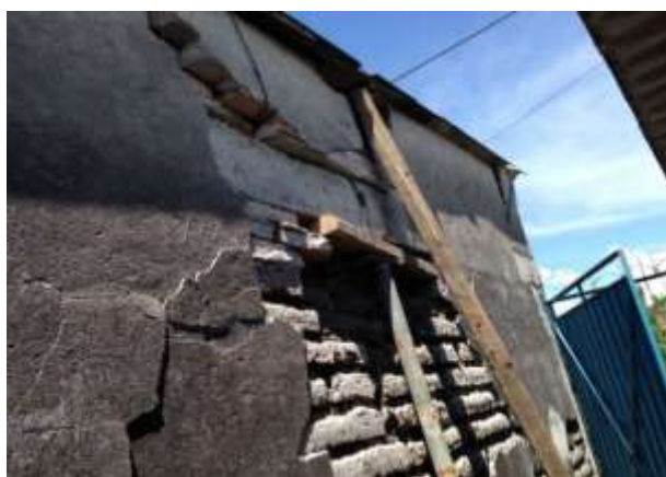
Figure 6 housing where the bending perpendicular to the plane of the adobe wall intensified by the structural failure of the enclosure is shown because the confined wall is not found and there is no effective distribution of the loads Source: Faculty of Architecture BUAP, 2017
