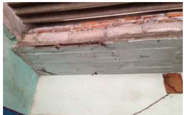
Figure 14 Interior view of the house of the image where reinforced concrete frames are integrated and rooms are added with other materials without taking care of the joints between one system and another Source: Faculty of Architecture BUAP, 2017
