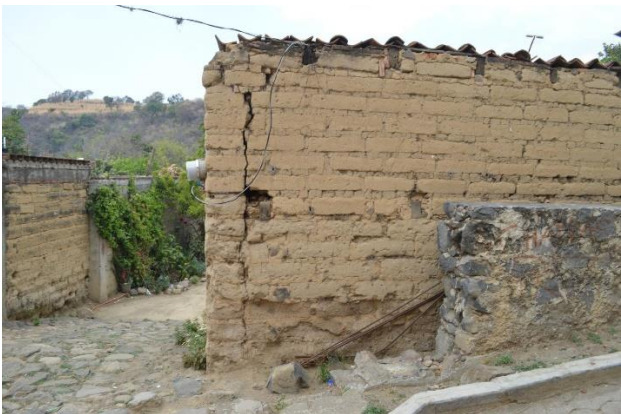
Figure 9 Flexion perpendicular to the plane in the unconfined corners of loose walls, or in corners not effectively connected with the transverse walls, caused by the earthquake of September 19, 2017
