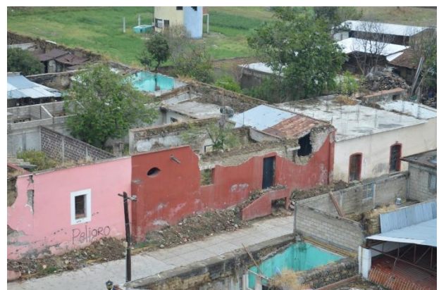
Figure 7 Aerial view of historic dwellings damaged by the earthquake of September 19, 2017 Source: Vázquez, August 2018
