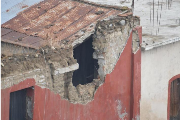
Figure 8 Bending perpendicular to the wall plane. Cracking in the intermediate height and additional vertical cracking, frequently occurs in long walls caused by the earthquake of September 19, 2017 Source: Vázquez, August 2018
