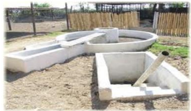
Figure 3 Fixed dome plant. Web image. F. Cut Problems biogas technology. Cuba, CUBASOLAR (No. 36, December 2006).
