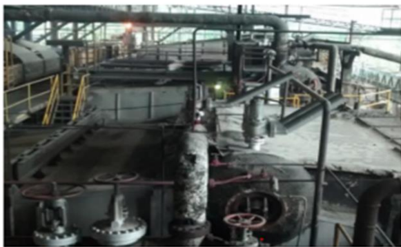
Figure 2 Top view of the dome of a modern bagasse boiler Source: Own elaboration
