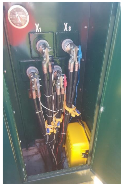
Figura 2 Three-phase HIOKI connection
