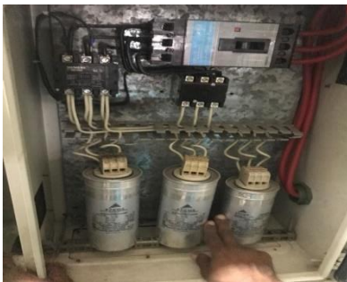
Figure 1 20 KVA capacitor bank in the company Hielo San Bartolo
