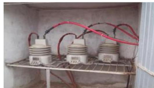
Figure 1 CT'S current transformers with weakened conductor and in poor conditions.
