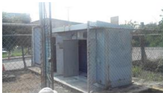
Figure 3 Set of switching substation and current transformers TC'S
