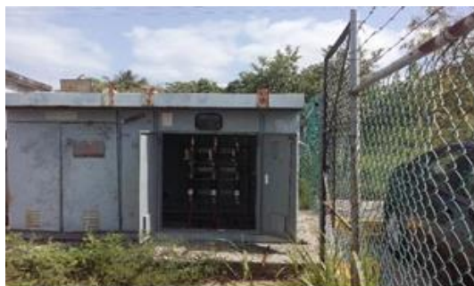
Figure 2 Switching station of the (UTSV) with hardware recently replaced and under maintenance.
