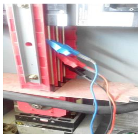
Figure 7 Connections for voltage detection of the power quality analyser equipment
