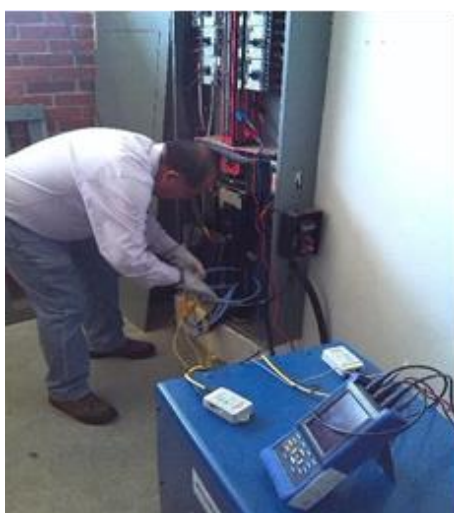
Figure 5 Inspection and analysis of power quality - in situ with hikoi 3197 equipment
