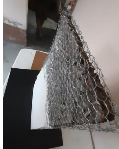
Figure 20 The figure shows the mesh that not only acts structurally, but also as a connection between panels
