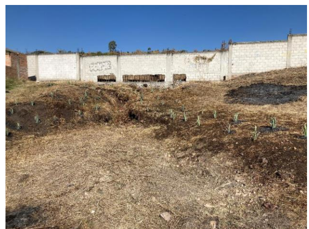
Figure 5 Conditions of the intervention site, where the runoff margins were cleaned and revegetated
