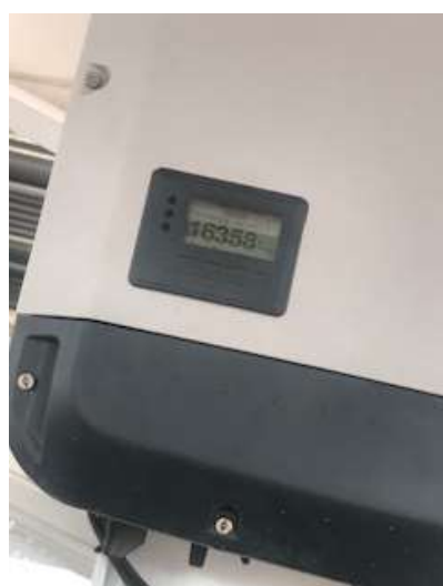
Figure 9 Inverter injecting power from PV modules 11:00 a.m Source. Own Elaboration
