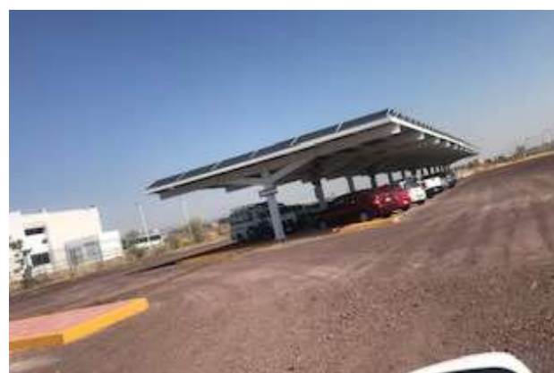
Figure 6 SFVI installed Source. Own Elaboration
