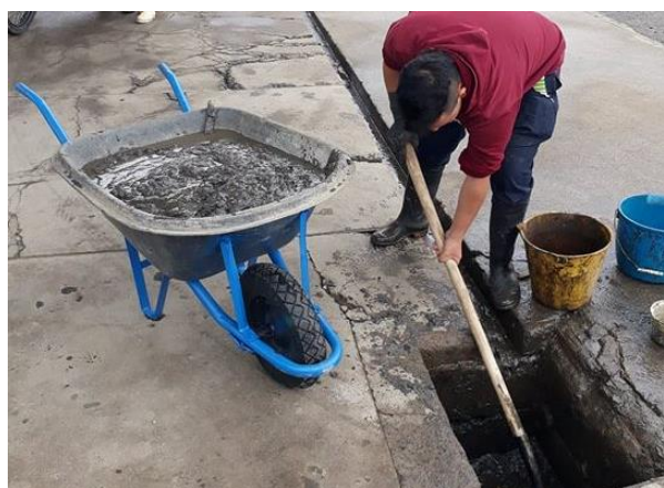
Figure 2 Extraction of sediments from the grease trap
