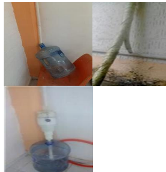
Figure 2 condensate water collection systems air conditioning chemical laboratory
