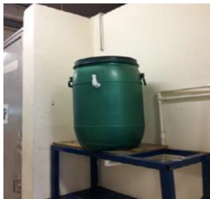
Figure 3 condensate water collection systems air conditioning electromechanical workshop Source: Own Elaboration
