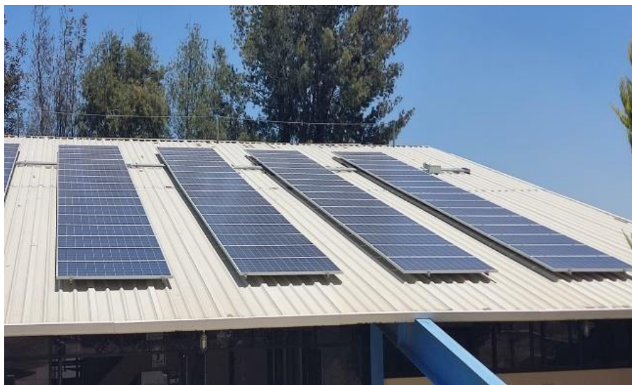
Figure 2.1 Photovoltaic power plant
