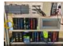
Figure 9 Siemens S7 1200 PLC Control Panel, HMI and Connections
