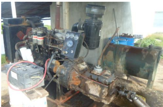
Figure 1 Current pumping in shrimp farm
