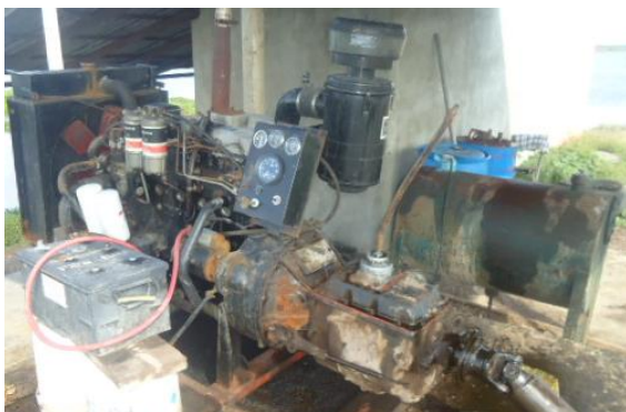
Figure 1 Current pumping in shrimp farm
