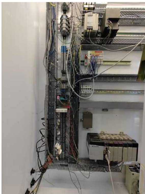
Figure 3 Cabinet with the connections between the robot and the PLC
