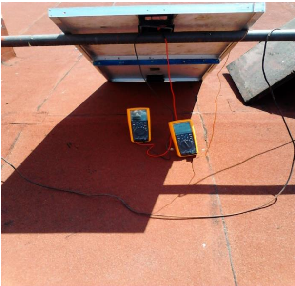
Figure 5 Measurement of electrical figure of merit of solar energy conversion
