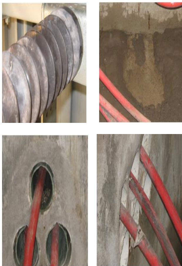
Figure 9 Damage in the electrical substations
