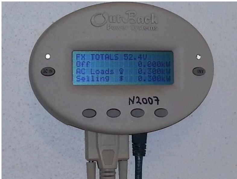
Fig. 5 UNISTMO Controller panel.
