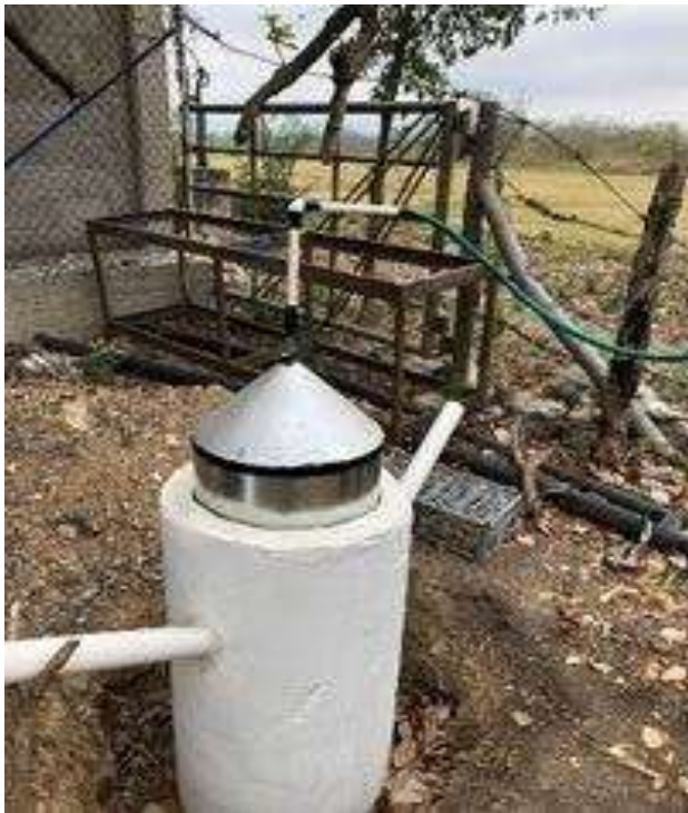
Figure 3 Placement of the floating hood Own Source
