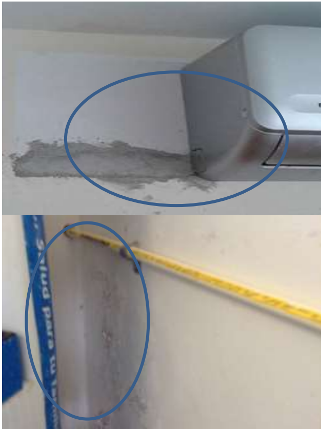
Figure 16 General damages in painting Source: Own
