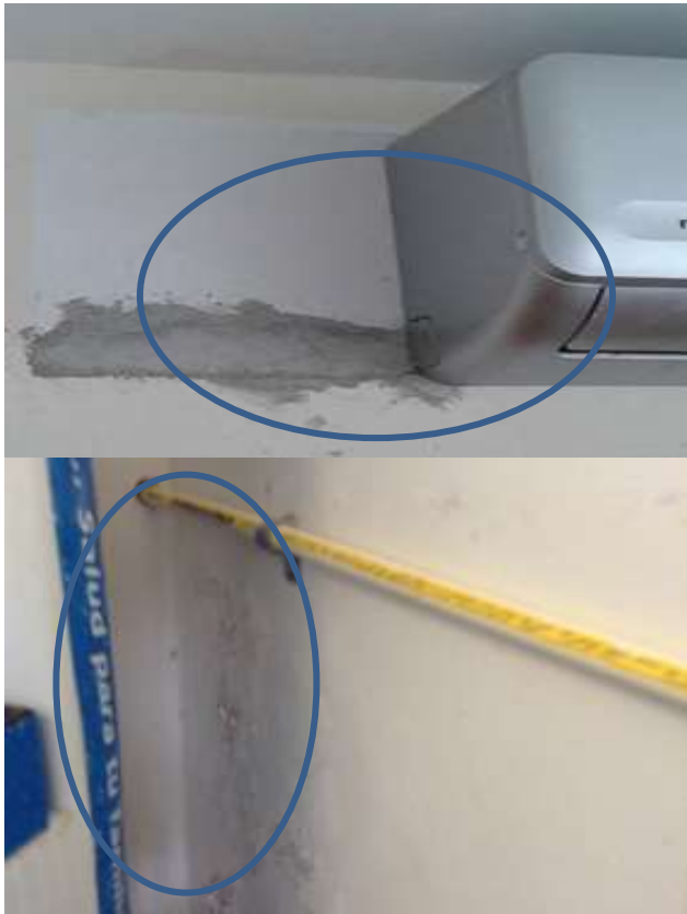
Figure 16 General damages in painting Source: Own
