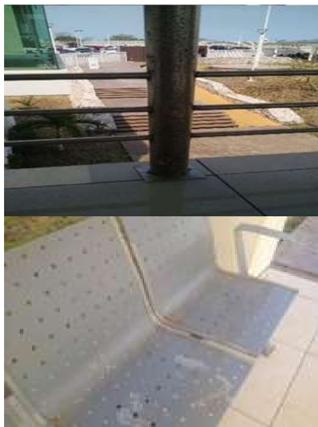
Figure 15 Corrosion in metal structures
